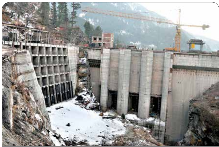
The first unit of the 4x200 mw Parbati Hydro Electricity Project, Stage-II, in Kullu District, Himachal Pradesh, was successfully spun at 3 pm on March 31 and further tests of the unit are in progress. The water of JiwanaNallah has been diverted into the main Head Race Tunnel through a Drop Shaft for this task. Subsequently, spinning and testing of other units are also to be achieved in a similar manner
